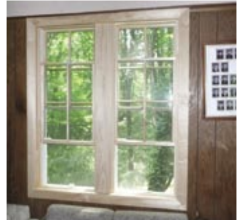
New Pella windows will add to appearance of the Lodge as well as reduce heating costs.
