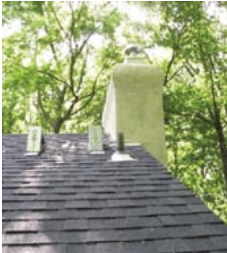
A view of new asphalt shingles and new stucco exterior of chimney
